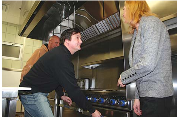
Tom Jankowski of Quality Stainless shows Shelly Mazur with the Farmers Market the new stove installed in the market's kitchen, while contractor John Spudich, far left, looks on.
